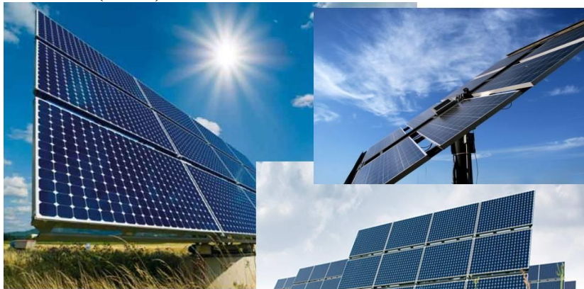
Fig 3. Solar Power Plant (PLTS)
